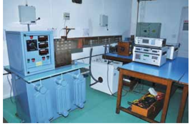
Fig. 2.6 The National Standard of AC High Current Ratio Measuring System upto 5000A/1A, 5A
