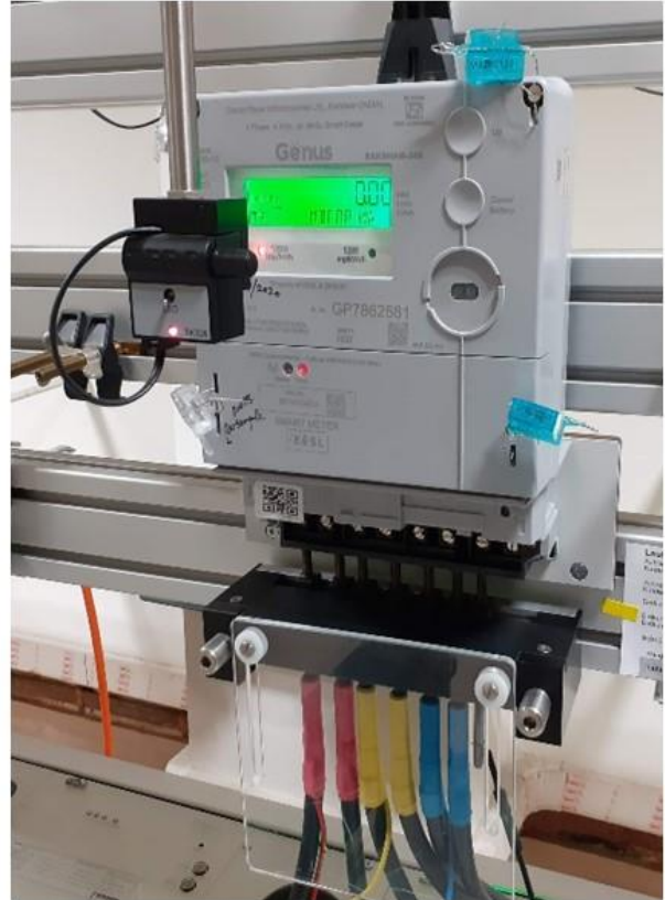
Testing of smart energy meter
