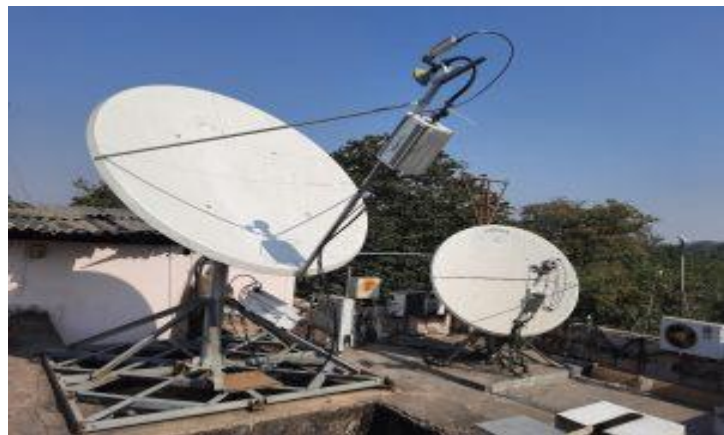
Outdoor portion of two VSAT's of 2.4m diameter dish antenna each at NPLI. Left one is being used for international link and the right one is used for domestic link
